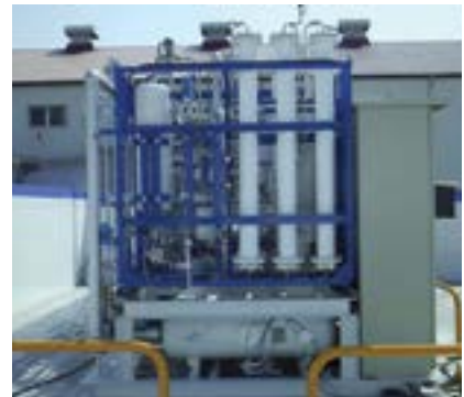
XEBEC 3200-G2 IN JAPAN Hydrogen Plant in Tokyo
