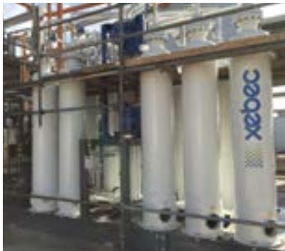
XEBEC 3200-G4 IN USA Ethylene cracker off-gas
